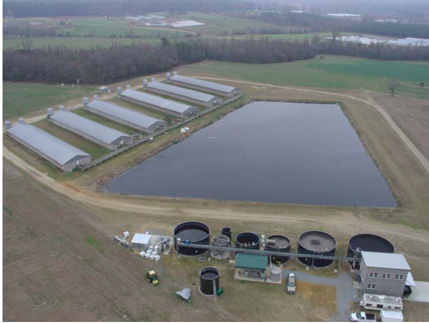
Figure 1: Super Soil on-farm treatment technology installed at Goshen Ridge farm in Duplin County, NC.
